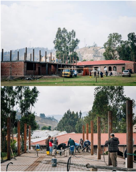
Eight months of construction including the Conovirus delays has produced 2 greatly needed buildings for classes.
